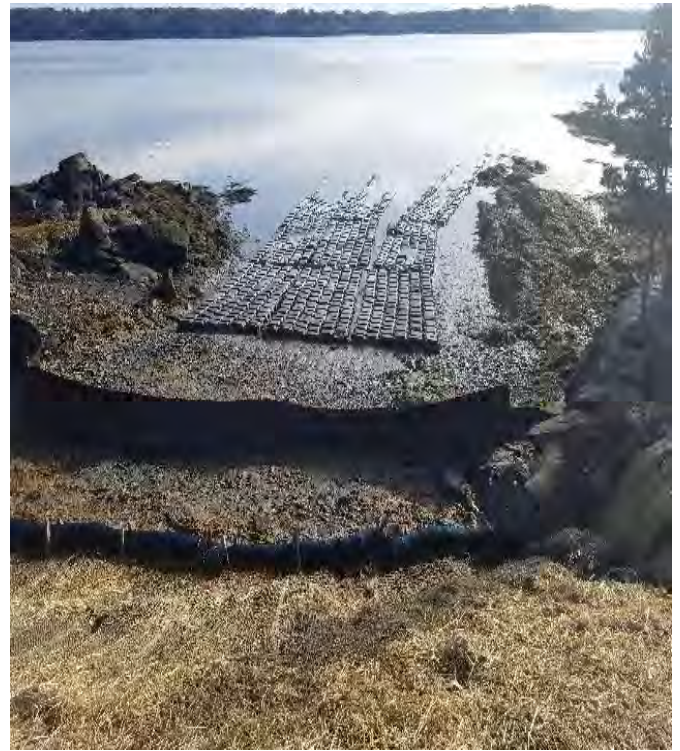
Fig 14: BMPs installed at toe of slope at Getchell property/west side of the Bay. Viewing east. (01-27-20).
