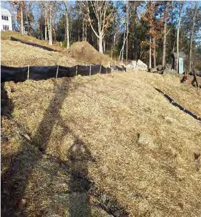
Fig 13: BMPs installed on slope at Getchell property/west side of the Bay. Viewing north. (01-27-20).
