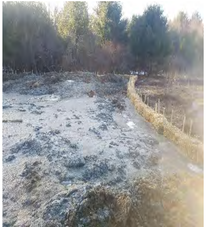
Fig 8: Soil spoils from drilling Str. 58 spread in turtle bed area between Strs. 48 and 49. Area is enclosed with straw bales. Turtle area is not Complete. Viewing west. (01-27-20).
