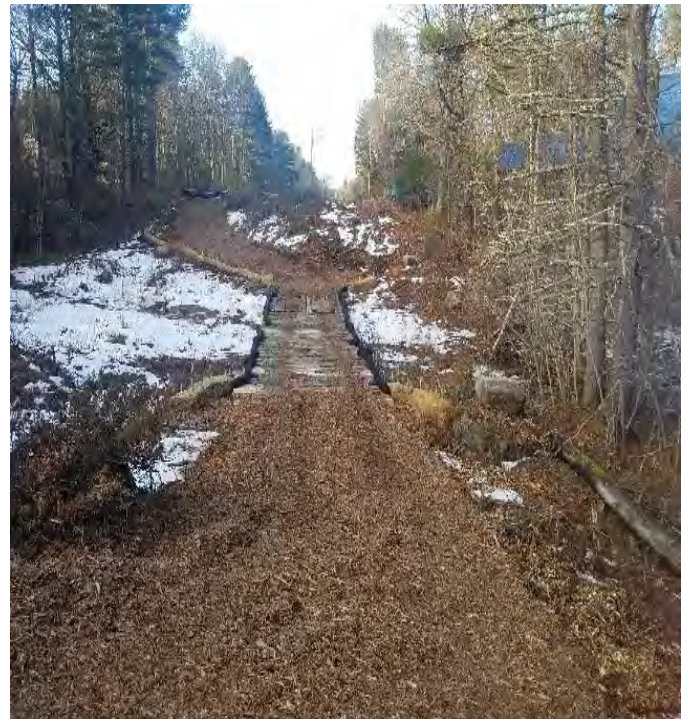
Fig 4: Access road through wetland DW9, between Strs. 65 and 66. Viewing west. Note stump grindings on slopes. (01-27-20).
