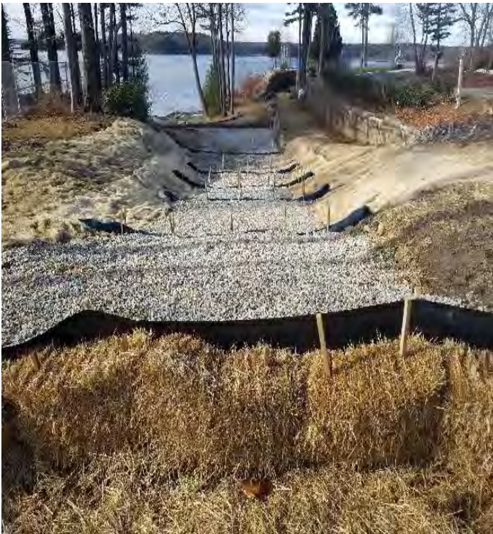
Fig 15: BMPs installed on slope at Gundalow landing/east side of the Bay. Viewing west. (01-27-20).
