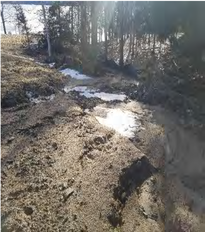
Fig 11: Rill on top of slope at Getchell property/west side of the Bay. Viewing southwest. (01-27-20).
