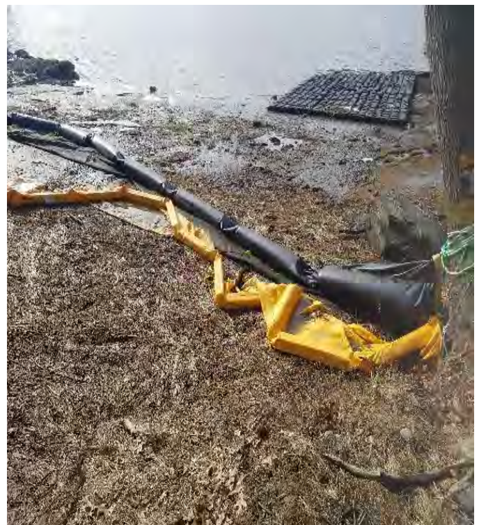
Fig 16: Turbidity barrier in intertidal zone at Gundalow landing/east side of the Bay. Viewing west. (01-27-20).
