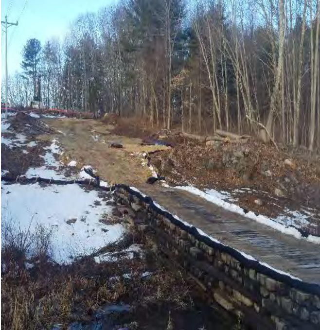
Fig 5: Access road to Str. 58 of off route 108. Bridge through wetland DW29. Viewing west. (01-27-20).
